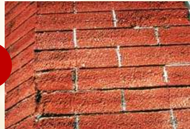
Bricks damaged from sandblasting (photos courtesy of NPS)
