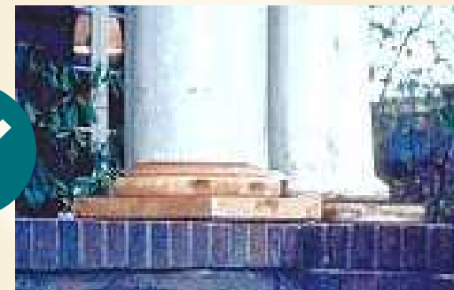
Replaced column base that matches looks and material (photos courtesy of NPS)
