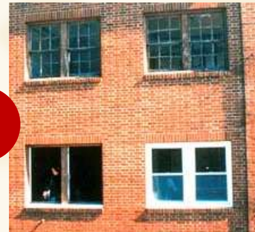
Replaced windows that damage historic character
