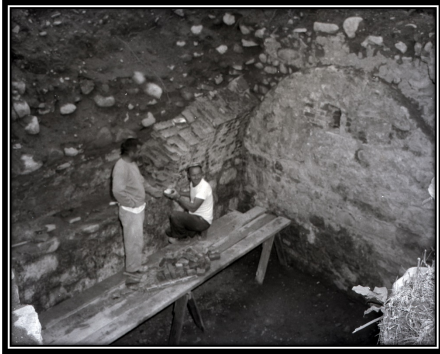
Figure 4-13. Photograph of the 1962 State of Maine Park Commission-funded restoration of the stone and brickwork of Fort George, in the south (southwest) bastion of the fort. Work pictured is on the vaulted brick magazine (Files of the Castine Historical Society).
