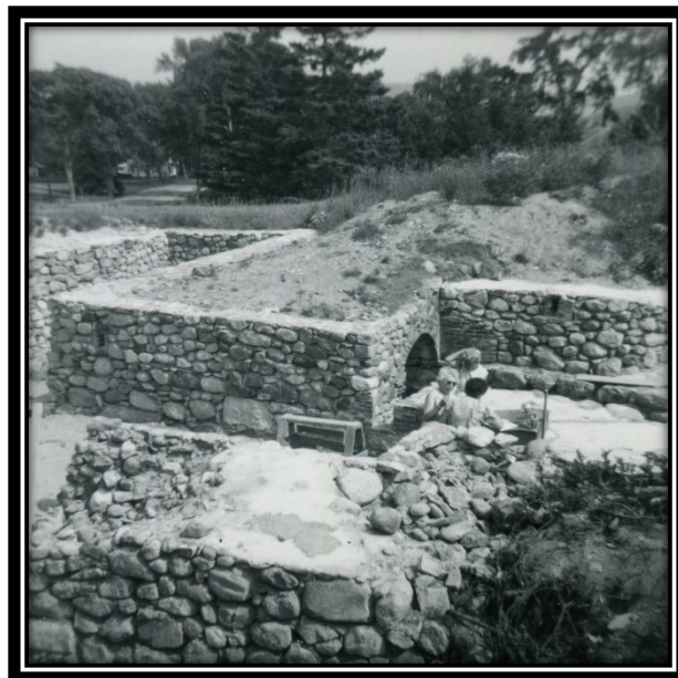
Figure 4-12. Photograph of the 1962 State of Maine Park Commission-funded restoration of the stone and brickwork of Fort George, in the south (southwest) bastion of the fort.
