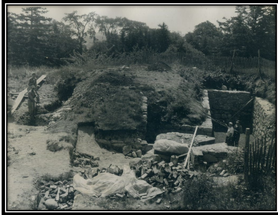
Figure 4-11. Photograph of the 1962 State of Maine Park Commission-funded restoration of the stone and brickwork of Fort George, in the south (southwest) bastion of the fort.
